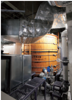
A water tank made of Japanese cypress is located in the machine room at the back of the parking lot.
